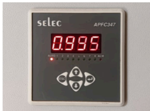
Fig 5.2 APFC relay after activation
