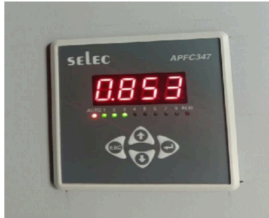
Fig 5.1 APFC relay before activation
